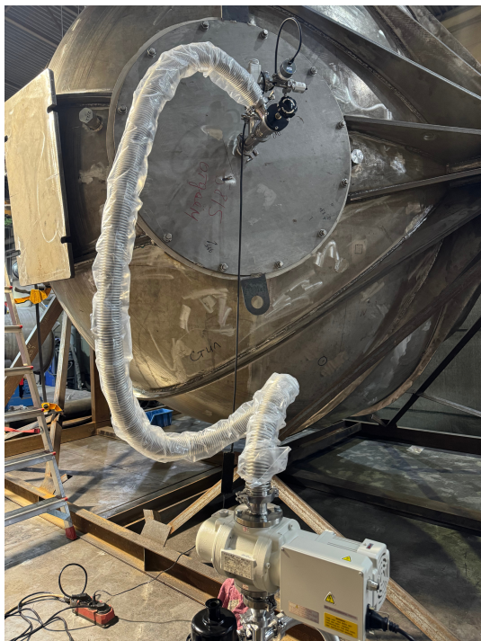
Figure 28 — Connecting line at the end assembly of a large vessel. Response assessment includes line length, cross-section and valve positions.
